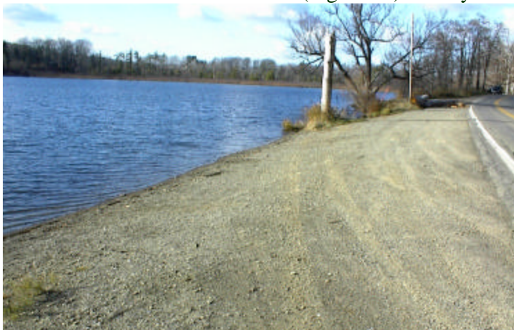
Figure 29. Degraded Lake Pleasant shoreline and State Route 1001, Lake Pleasant Road
