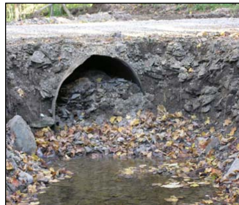
An inadequately designed culvert and endwall from a Buck Run tributary filled with sediment after a flood in 2004.
